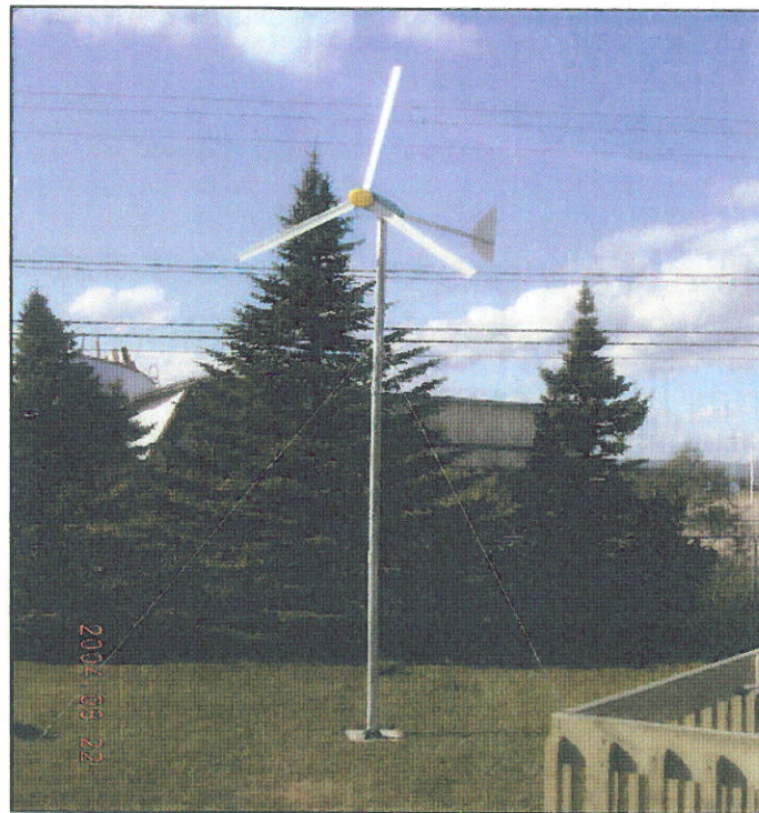
Step 13 Secure wires & connect to Batteries & Controller
